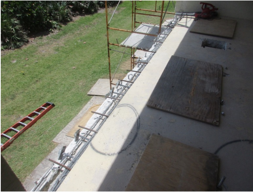
View of slab edge excavations completed on the Unit 313 balcony south end and reinforcing steel install in progress
