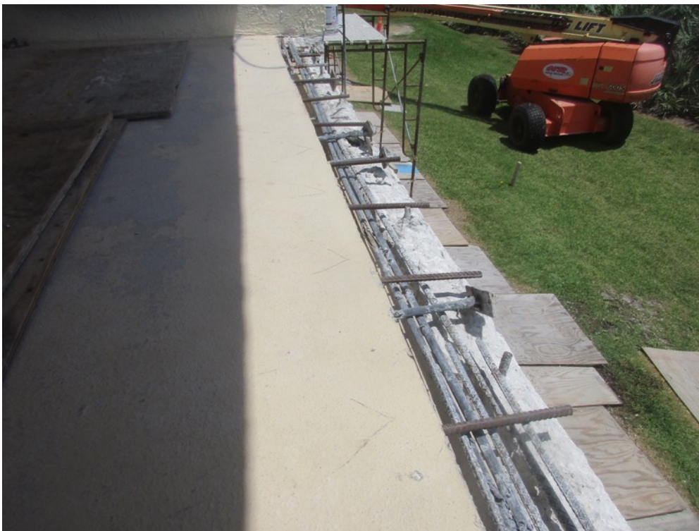
View of slab edge excavations completed on the Unit 313 balcony north end and reinforcing steel install in progress
