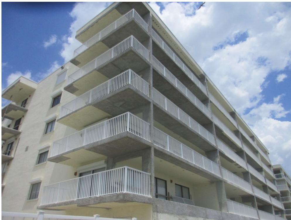
View of handrail installations wrapping up on the building 2 northeast corner 04 stack balconies
