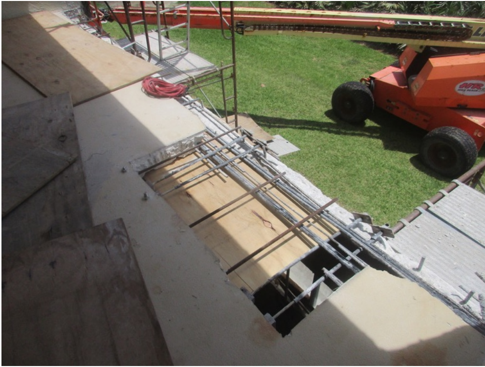
View of slab edge and full depth excavations completed with reinforcing steel install in-progress on the Unit 312 balcony north end
