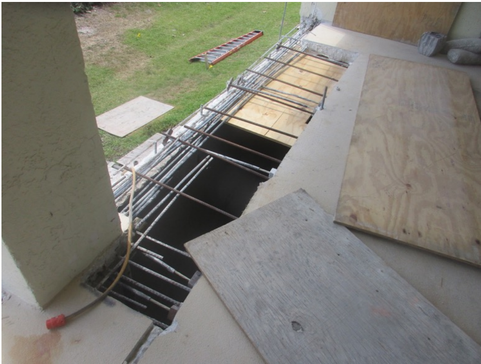
View of slab edge and full depth excavations completed with reinforcing steel install in-progress on the Unit 312 balcony south end
