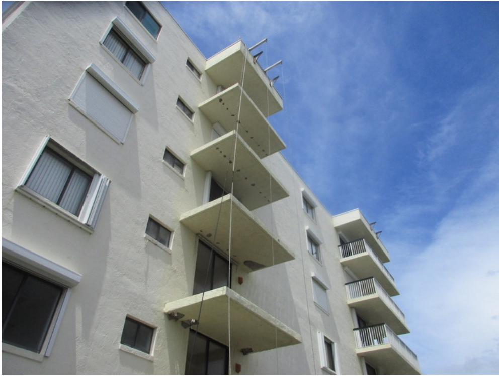
View of handrails removed from the 04 stack south side balconies with PT lock-off excavations in-progress
