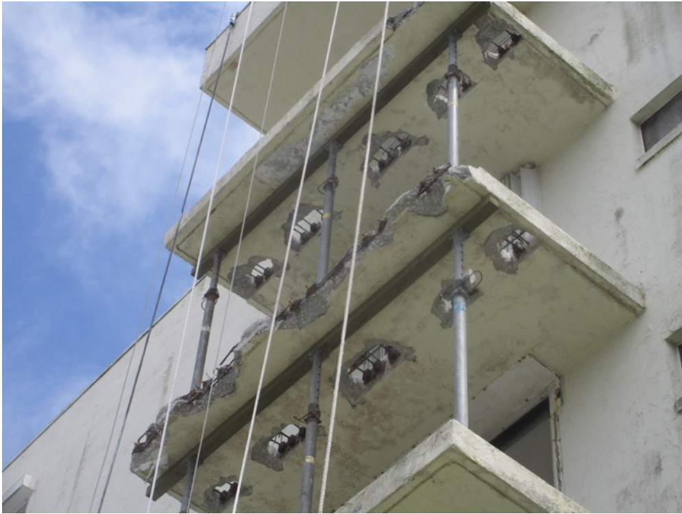
View of PT cables locked-off on the Unit 141 and 151 north side balconies
