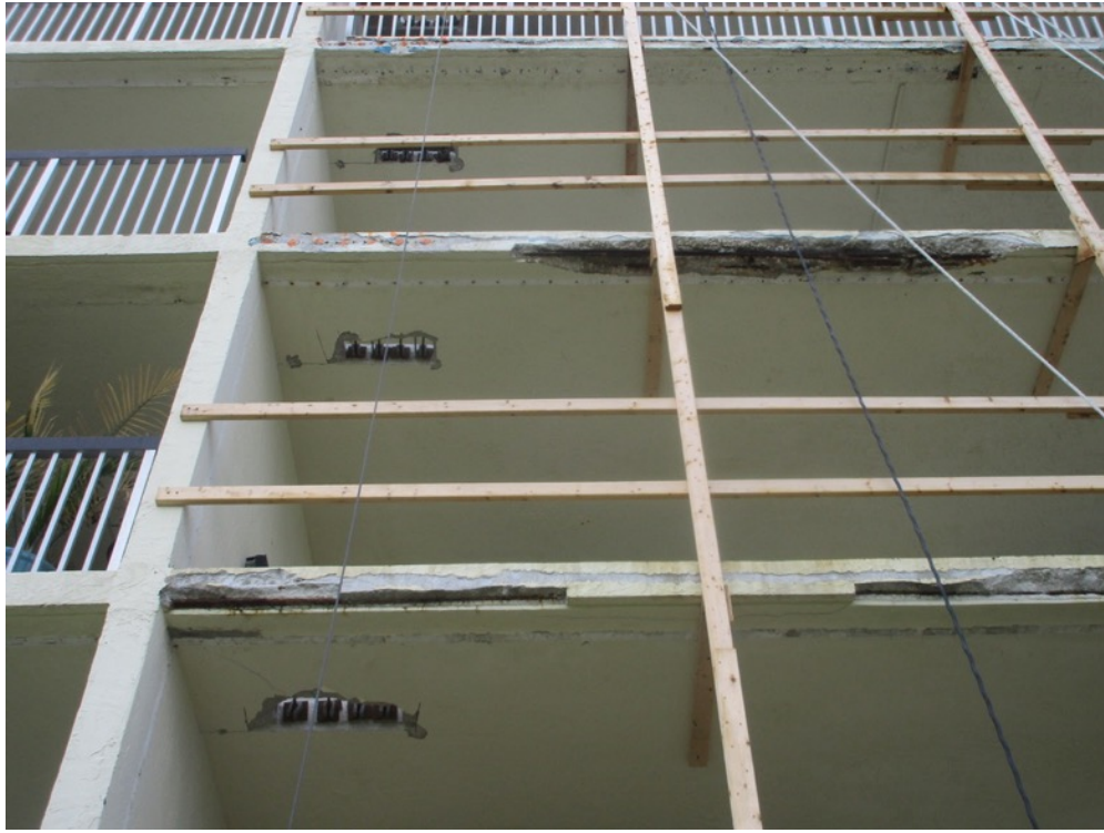
View of PT cable lock-offs installed on the 01 stack east elevation
