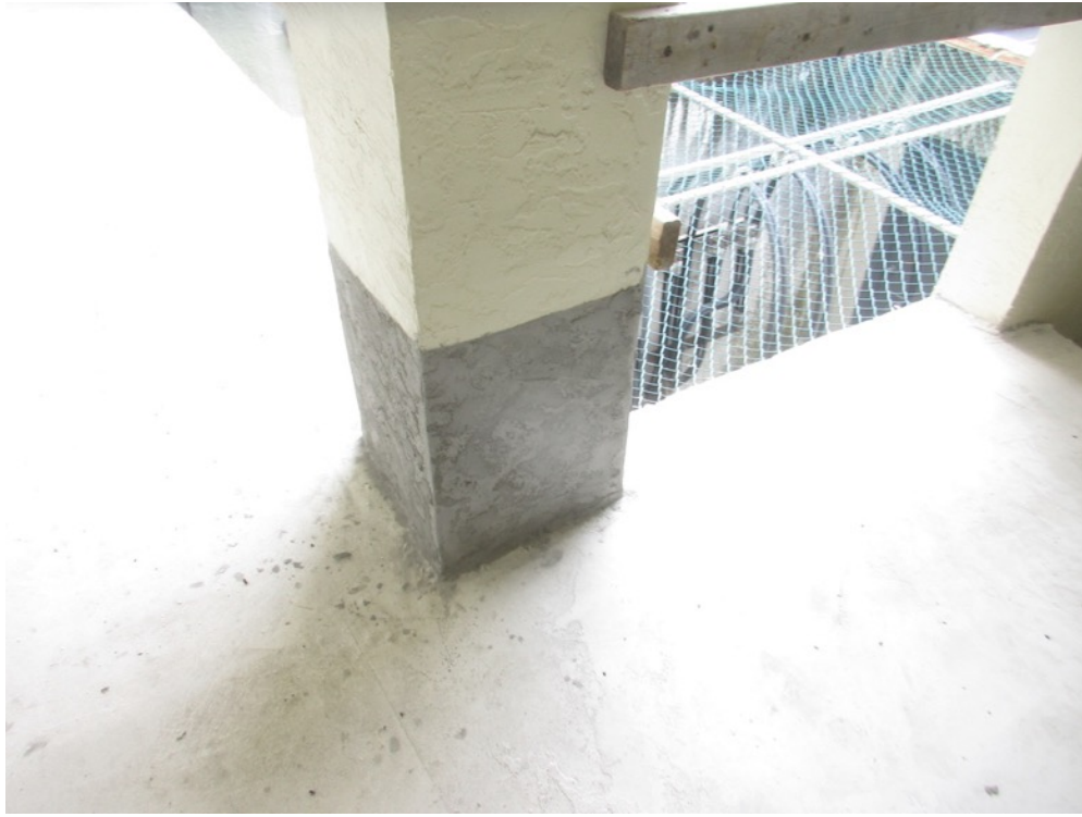
View of stucco finish applied to column repair outside Unit 211 on the walkway
