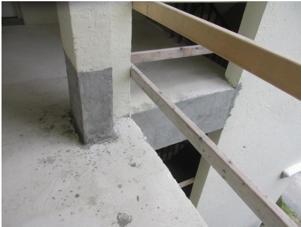
View of stucco finish applied to column and slab edge repair outside Unit 234 on the walkway
