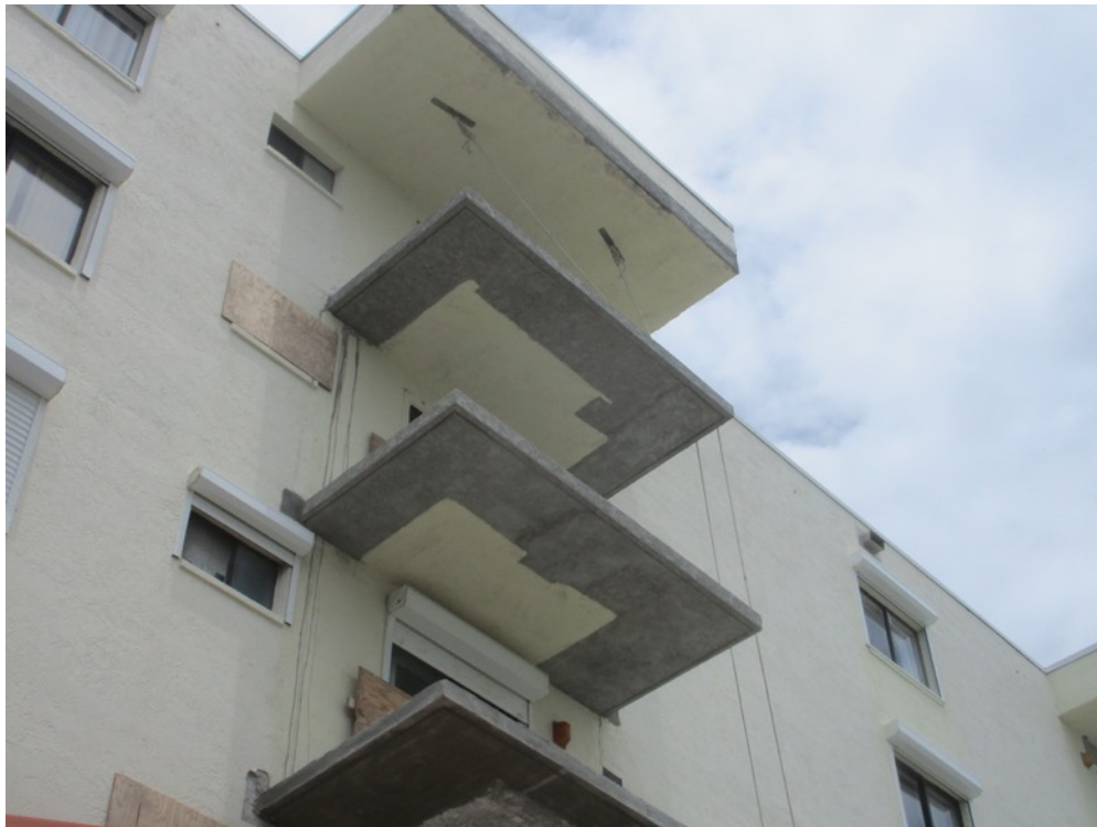
View of stucco finish applied to repaired areas on the Unit 244 and 254 SW kitchen balconies
