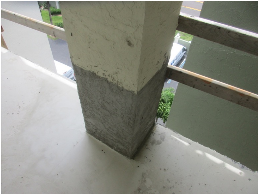
View of stucco finish applied to column repair outside Unit 243 on the walkway
