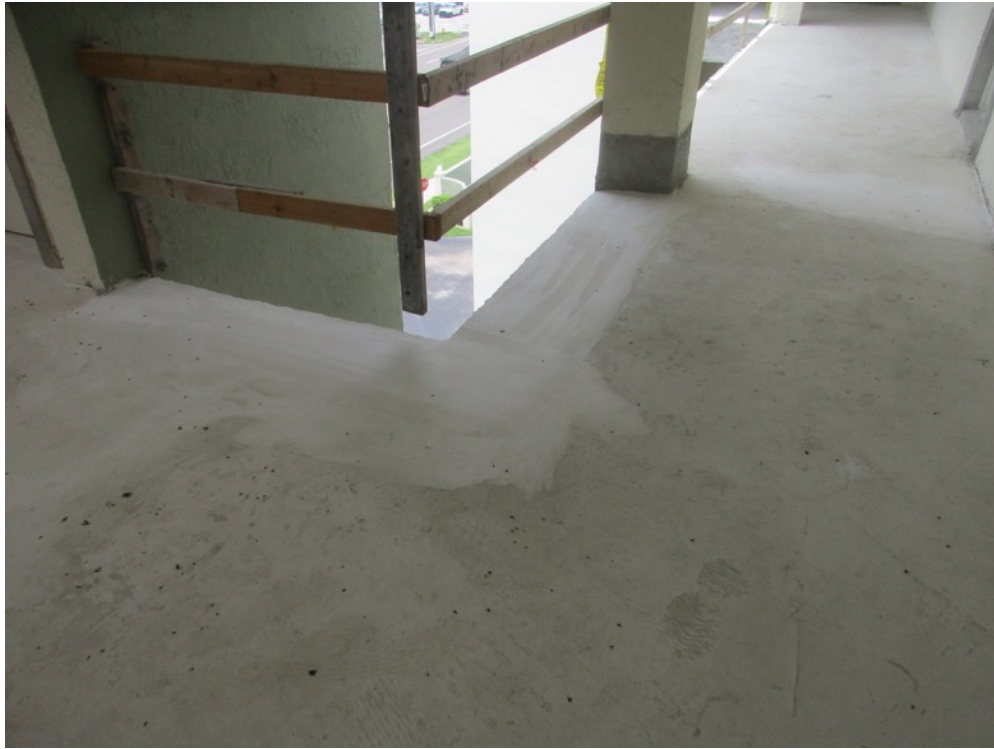
View of final surface profiling completed on the 5 th floor walkway elevator area
