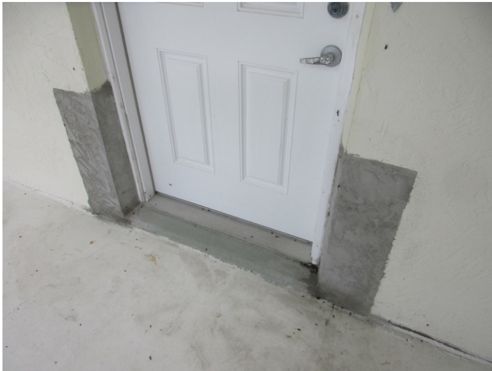
View of stucco finish applied to column repairs at the Unit 252 walkway entry door
