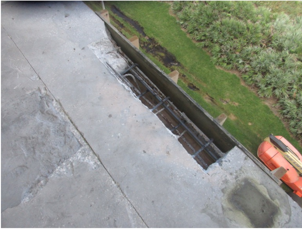
View of slab edge excavation completed with forms constructed and reinforcing steel set on the Unit 154 balcony
