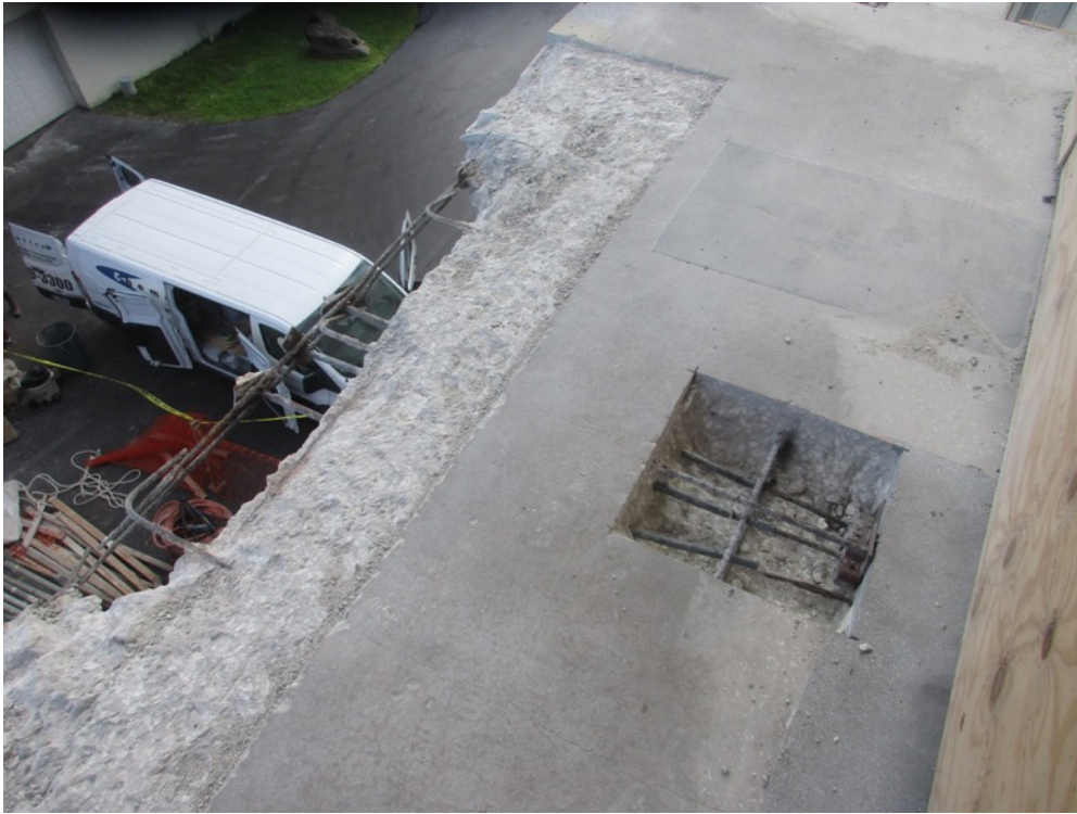
View of north-south PT cables locked-off with slab edge demo in-progress on the Unit 134 balcony south side
