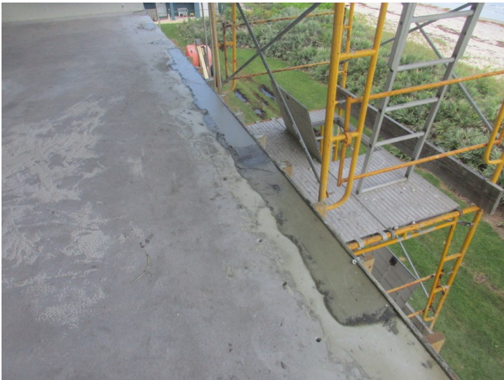
View of slab edge repair cast back on the Unit 134 balcony east side
