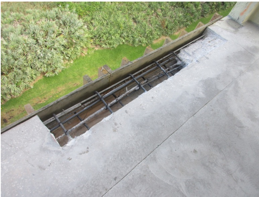
View of additional slab edge excavation completed with forms constructed and reinforcing steel set on the Unit 154 balcony
