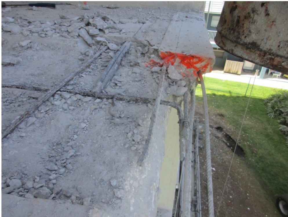
View of excavations in-progress on the Unit 132 balcony where a band of east-west cables begins and will require lock-offs to finish demo
