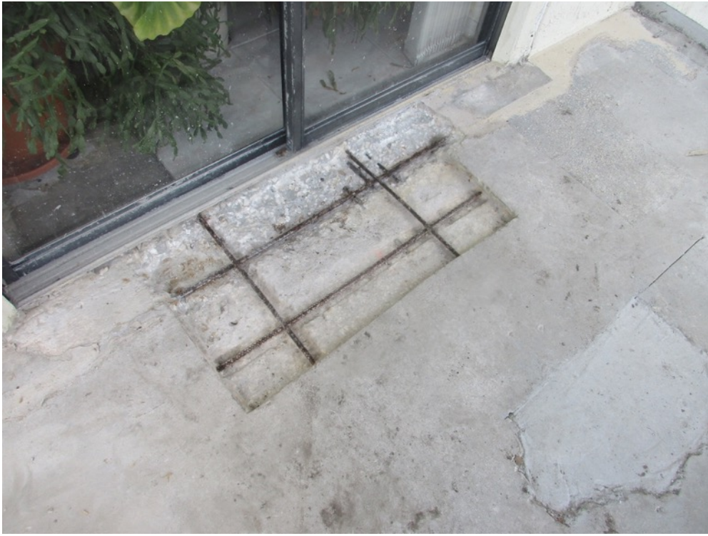
View of remaining surface excavations completed on the Unit 141 north side balcony
