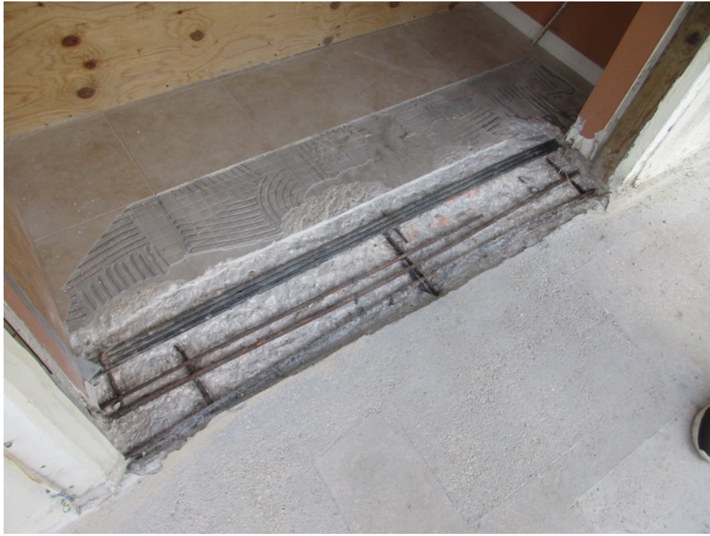
View of interior surface excavations completed on the Unit 111 north side balcony
