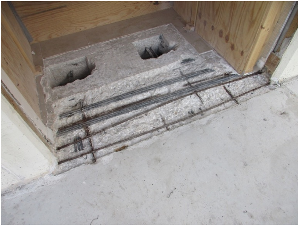
View of interior surface excavations completed on the Unit 121 north side balcony
