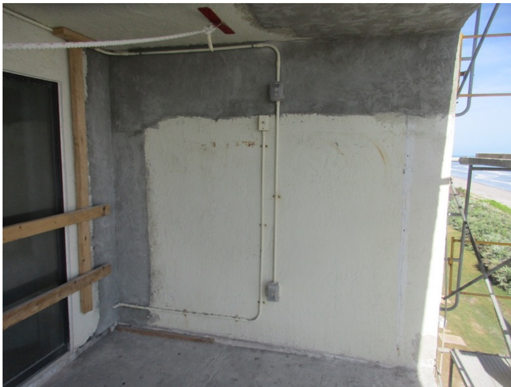
View of stucco finish applied to repaired areas on the Unit 232 north wall
