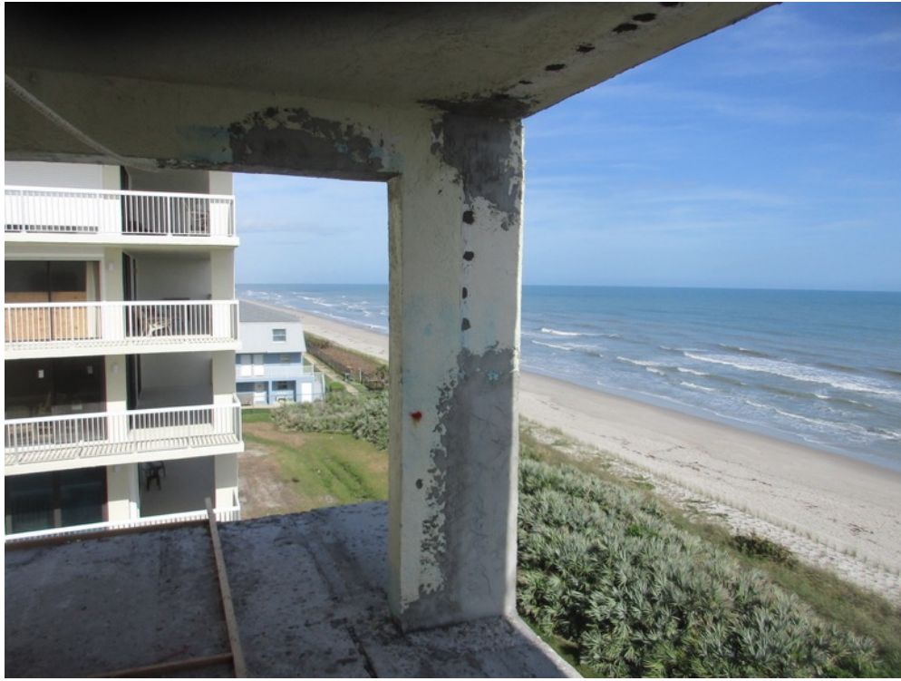
View of stucco finish applied to column repair on the Unit 241 balcony
