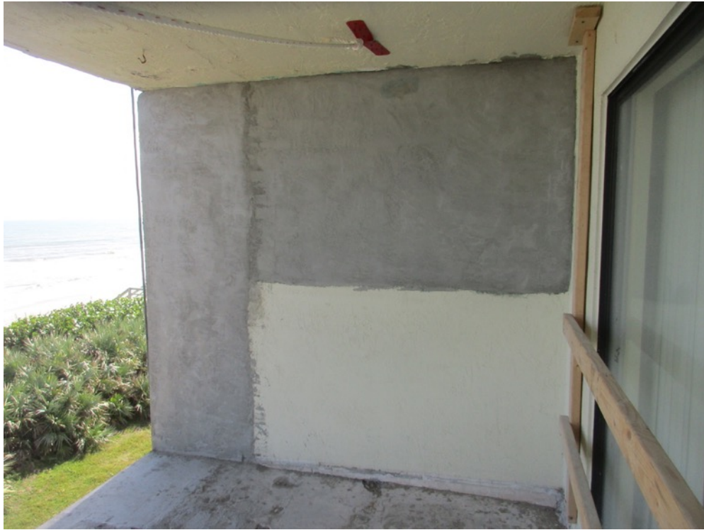
View of stucco finish applied to repaired areas on the Unit 222 south wall
