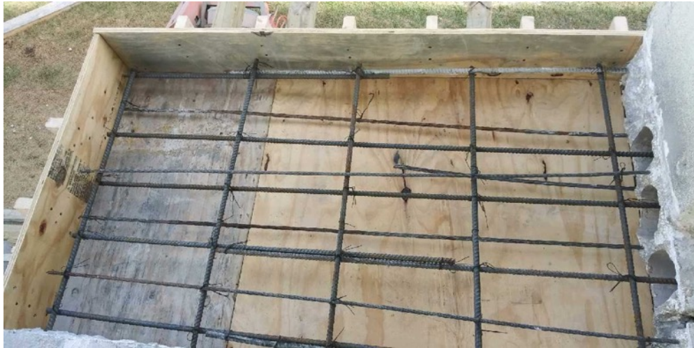
View of forms constructed with reinforcing steel set on the Unit 211 northeast corner
