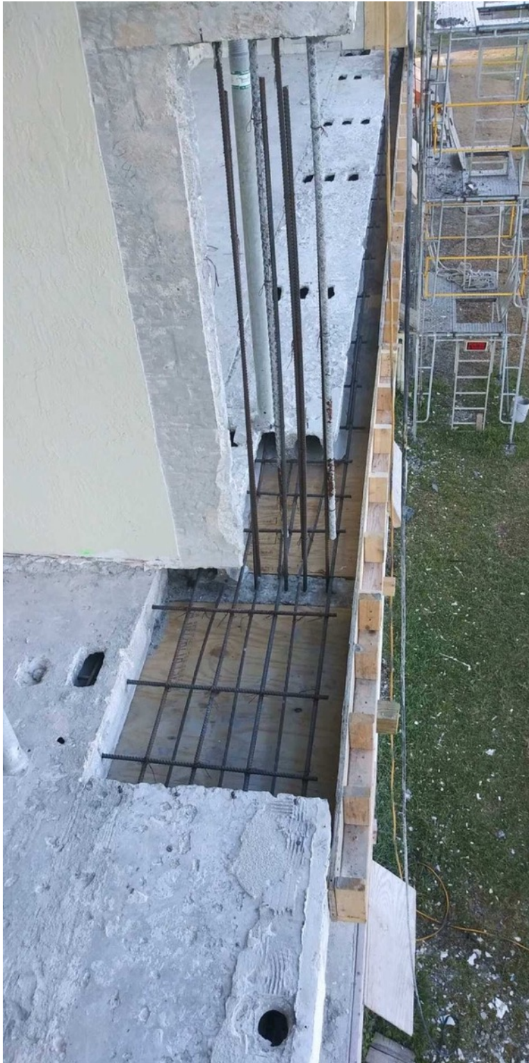
View of reinforcing steel set with formwork in-progress on the Unit 222/223 column and slab edge repair
