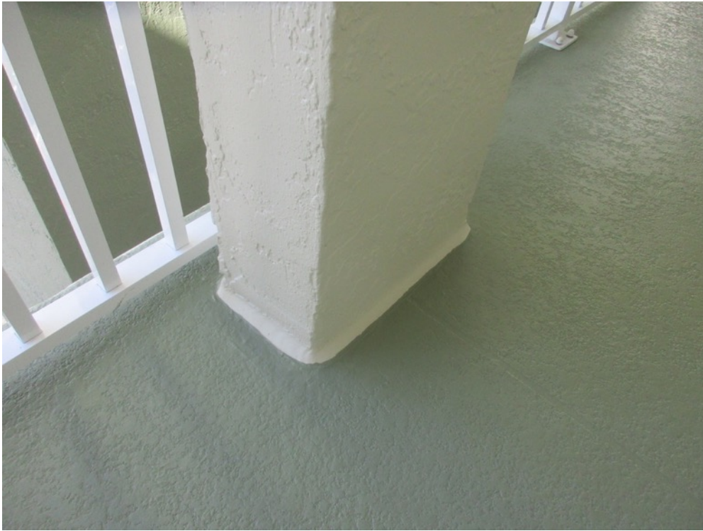
View of polyurethane cant bead tooled to column perimeter with cut-in completed on the 4 th floor walkway
