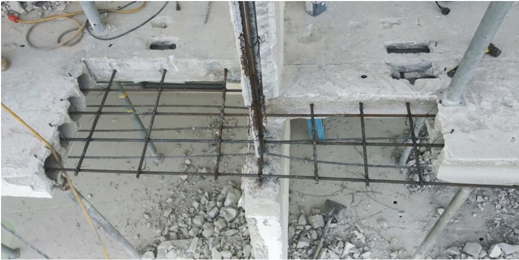
View of excavations wrapping up on the Unit 222/223 balcony divider column and hollow-core slab with reinforcing steel placement in-progress
