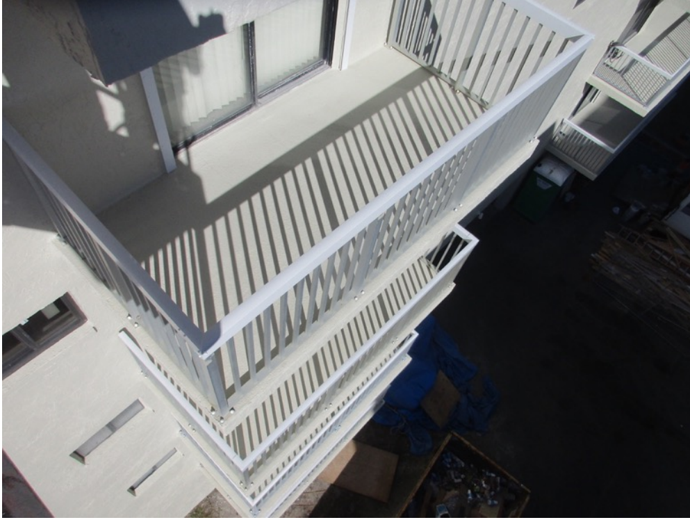
View of handrail top caps painted with deck coatings applied on the 04 kitchen stack balconies
