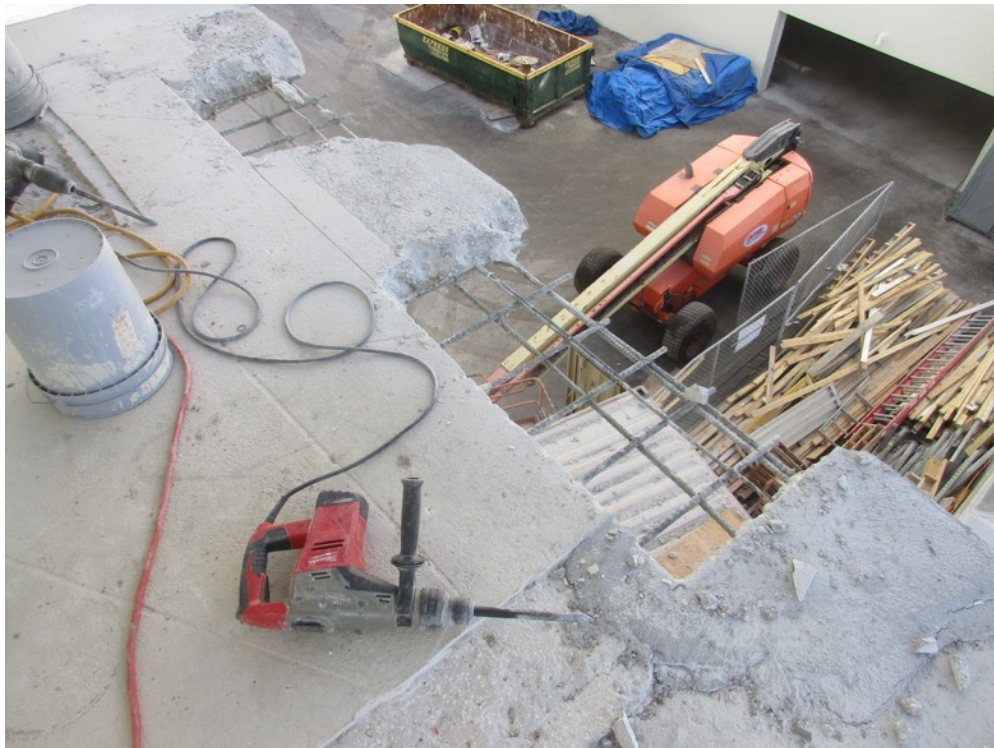
View of additional full depth/slab edge excavations in-progress on the Unit 231 balcony
