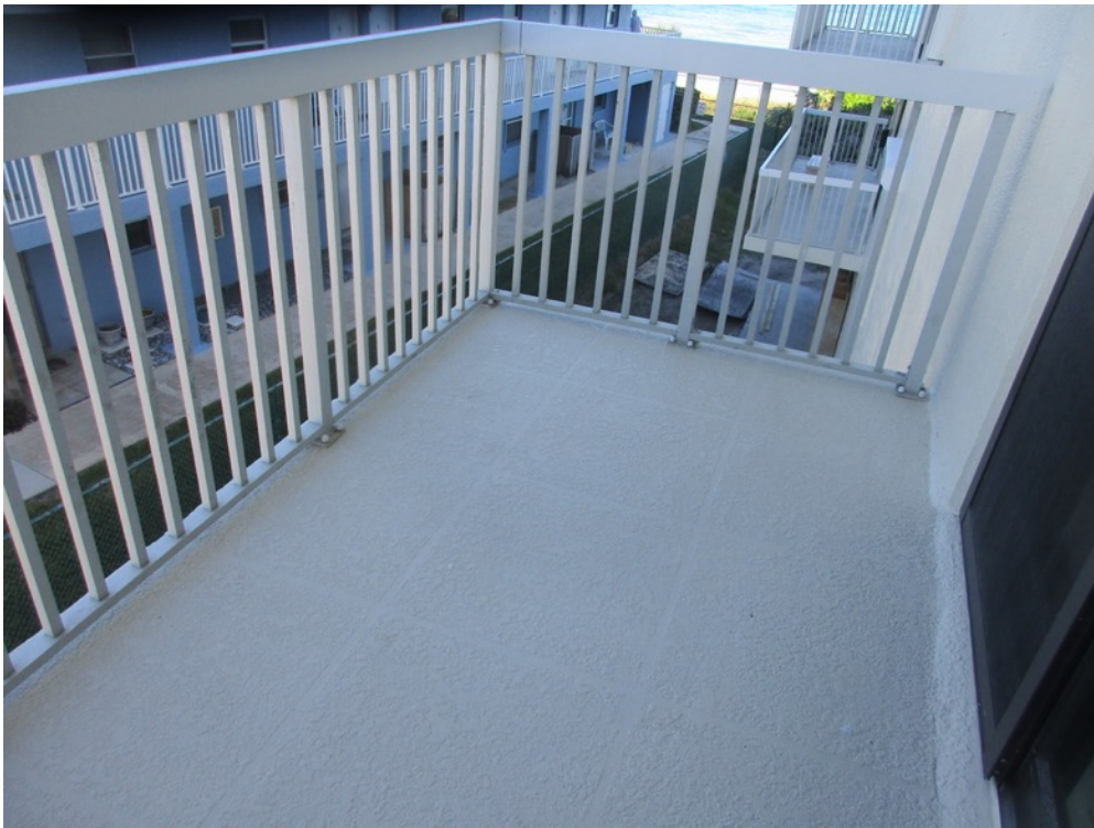
View of handrail top cap painted with deck coatings applied on the Unit 121 kitchen stack balcony
