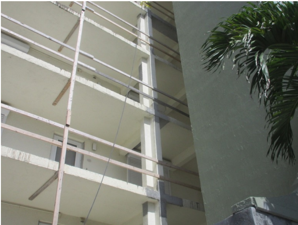
View of stucco finish applied to slab edge/column junctures on the north side walkways
