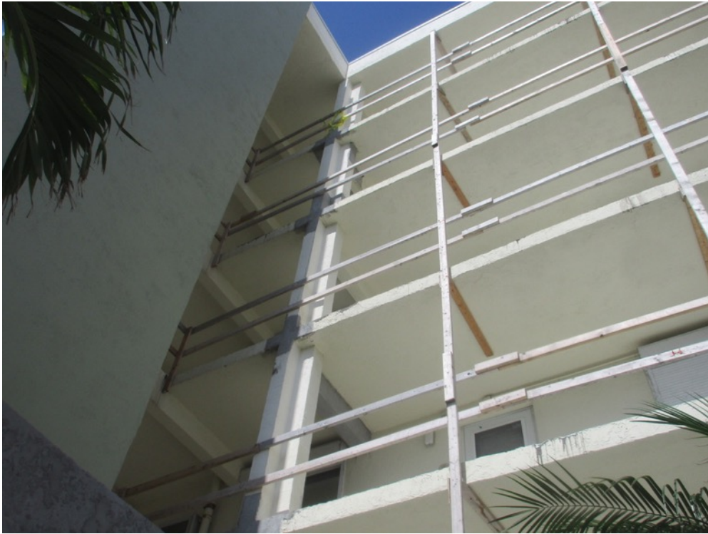
View of stucco finish applied to slab edge/column junctures on the south side walkways
