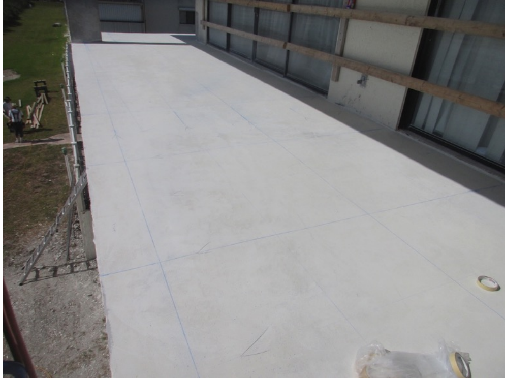
View of tile pattern grout line taping in-progress on the Unit 224 balcony deck
