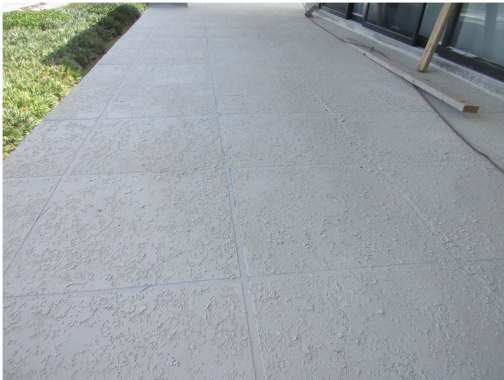
View of knockdown texture applied on the Unit 234 balcony deck with surface preparation sanding in-progress
