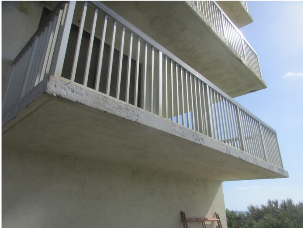
View of stucco removed from the Unit 314 slab edge where PT grout pockets have been covered by previous repairs
