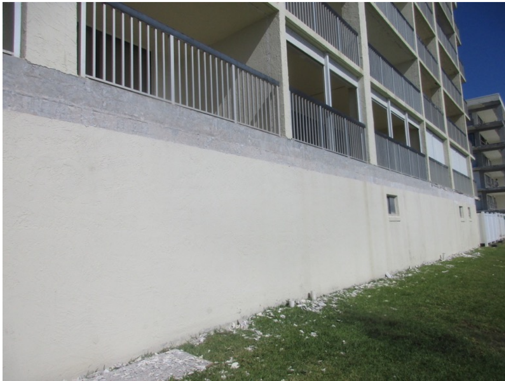
View of stucco removed from the building 3 east elevation 1 st floor slab edges where PT grout pockets have been covered by previous repairs
