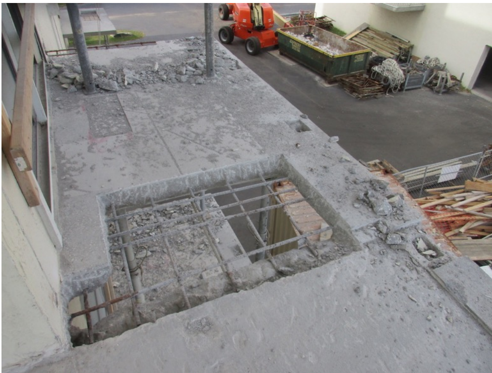
View of full depth excavations in-progress on the Unit 221 corner balcony north elevation
