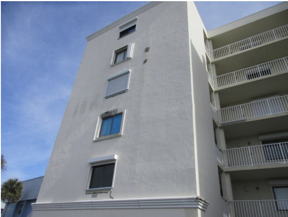
View of window header and stucco repairs completed on the 401 building west elevation shearwall north end
