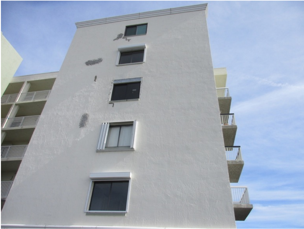
View of stucco repairs completed on the 401 building west elevation shearwall south end
