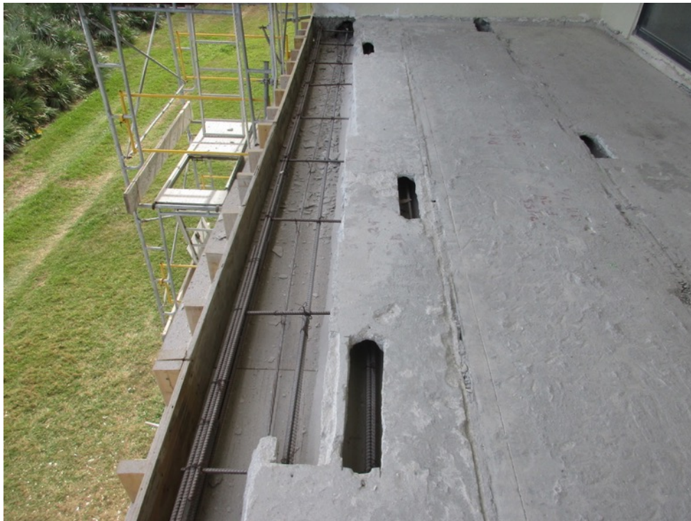
View of reinforcing steel placement in-progress on the Unit 221 balcony slab edge repair
