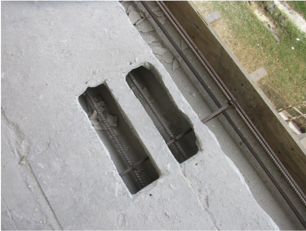
View showing #5 rebar set north-south in hollow-core cells on the Unit 221 balcony slab edge repair with east-west #4 rebar tied in
