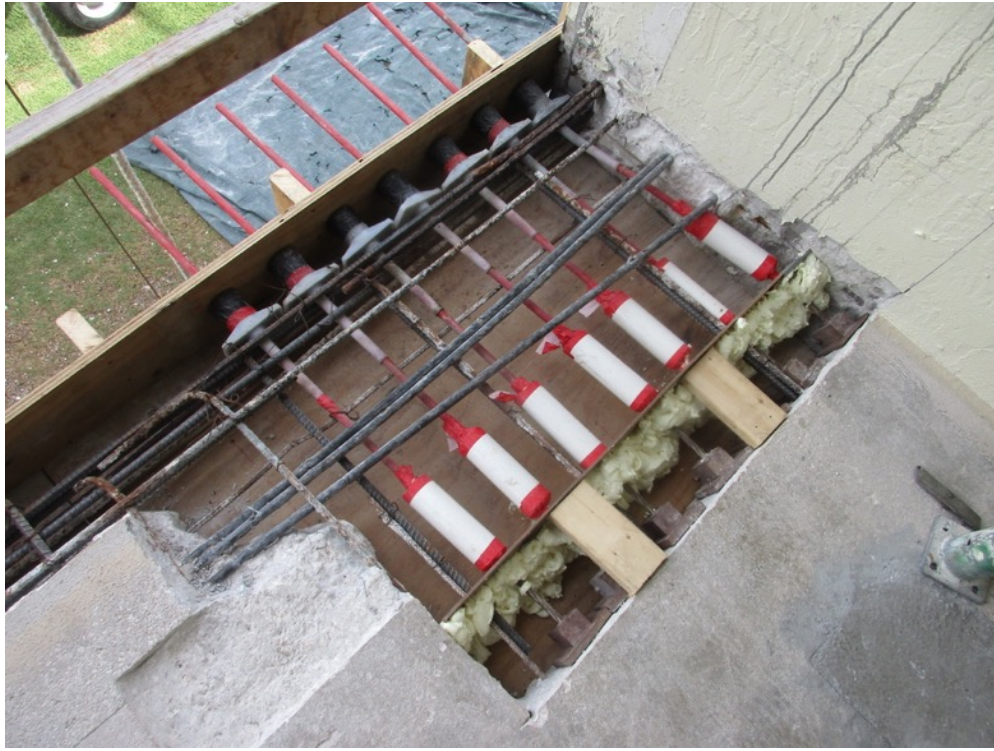
View of PT splice chucks/anchor heads installed on the Unit 121 south end band of 7 east-west cables
