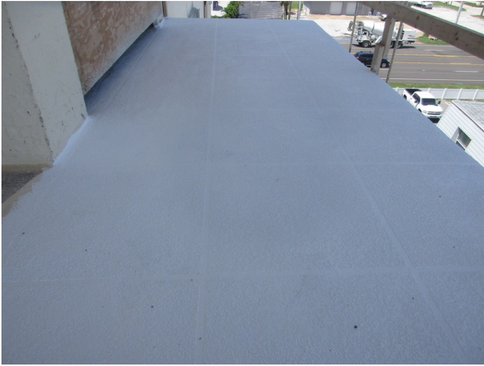
View of knockdown texture applied on the Unit 151 corner balcony north elevation
