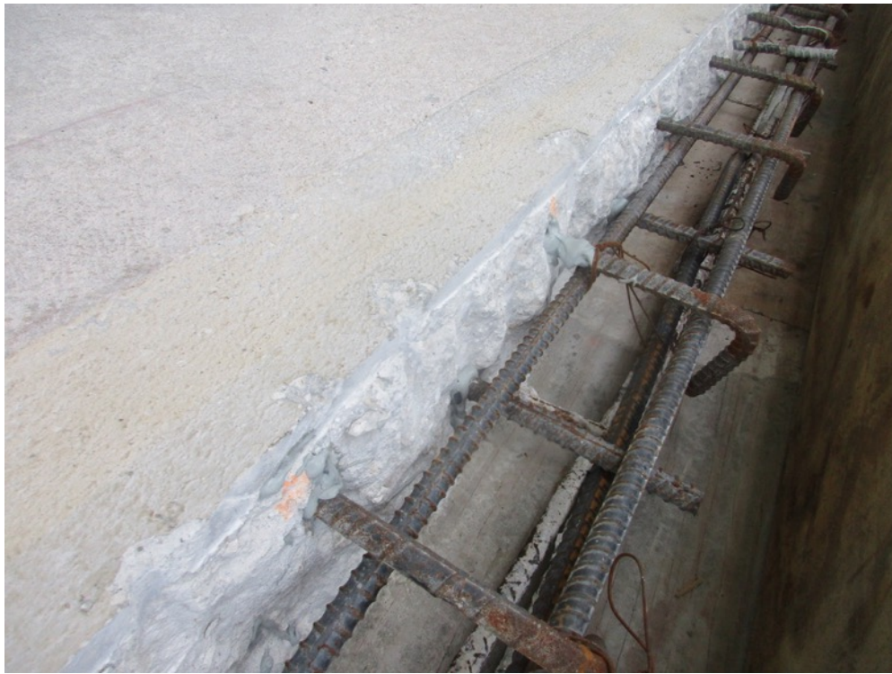
View of #5 rebar doweled-in/epoxy set on the Unit 121 east elevation slab edge
