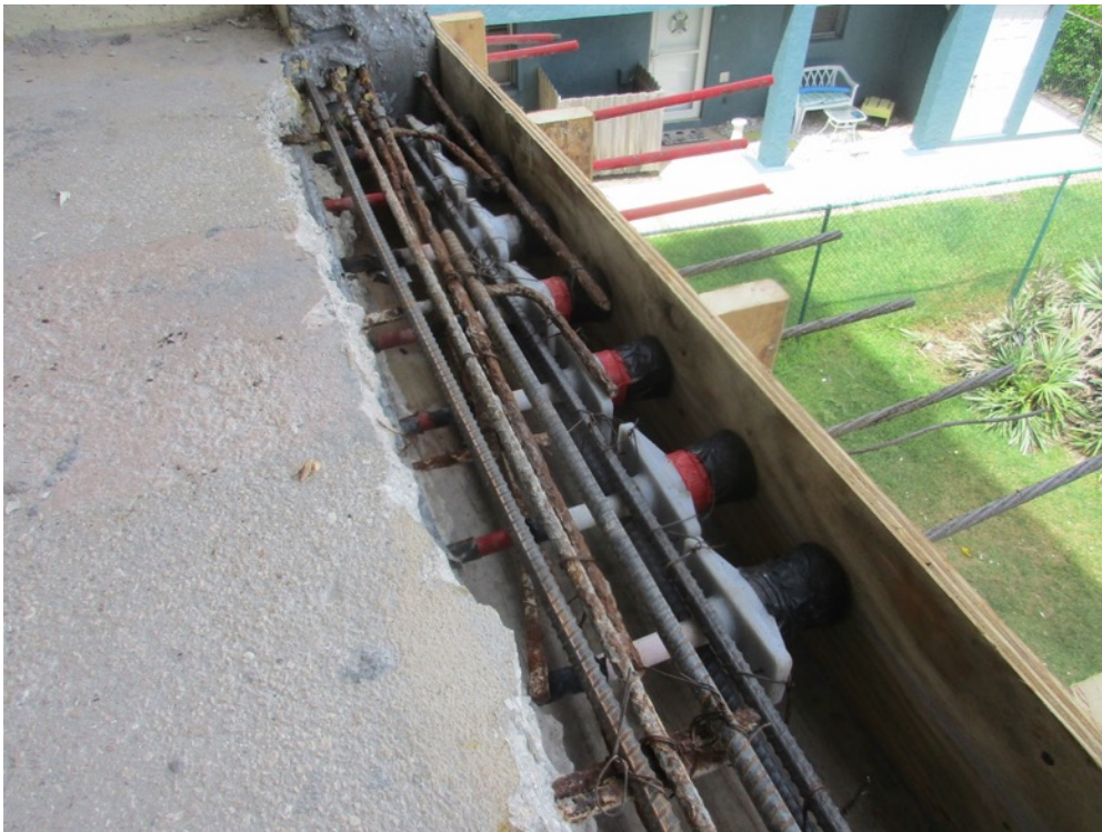
View showing PT anchor heads installed on the Unit 121 north band of 9 east-west cables
