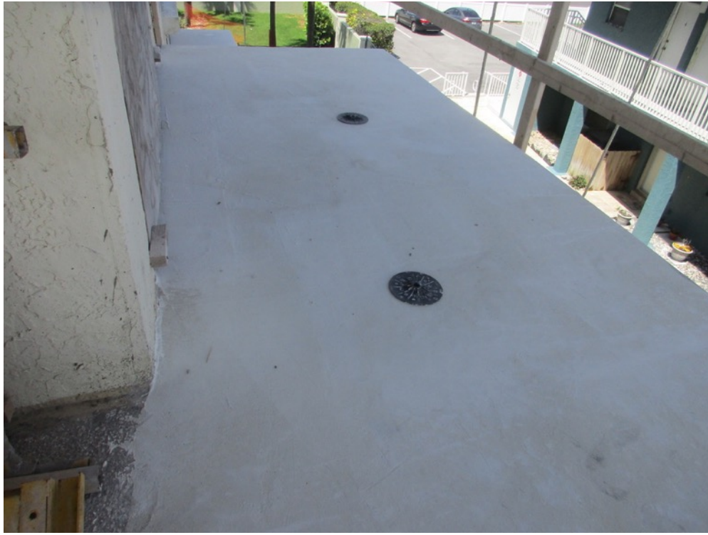
View of skim coats applied on the Unit 121 corner balcony north elevation
