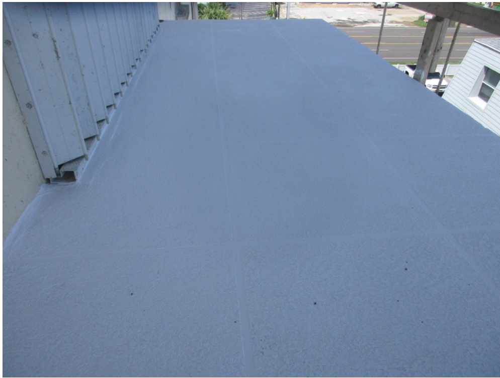
View of knockdown texture applied on the Unit 141 corner balcony north elevation
