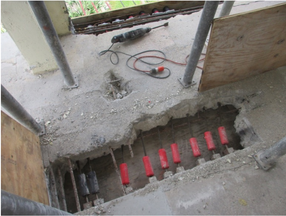
View of PT splice chucks/anchor heads installed on the Unit 121 north band of 9 east-west cables
