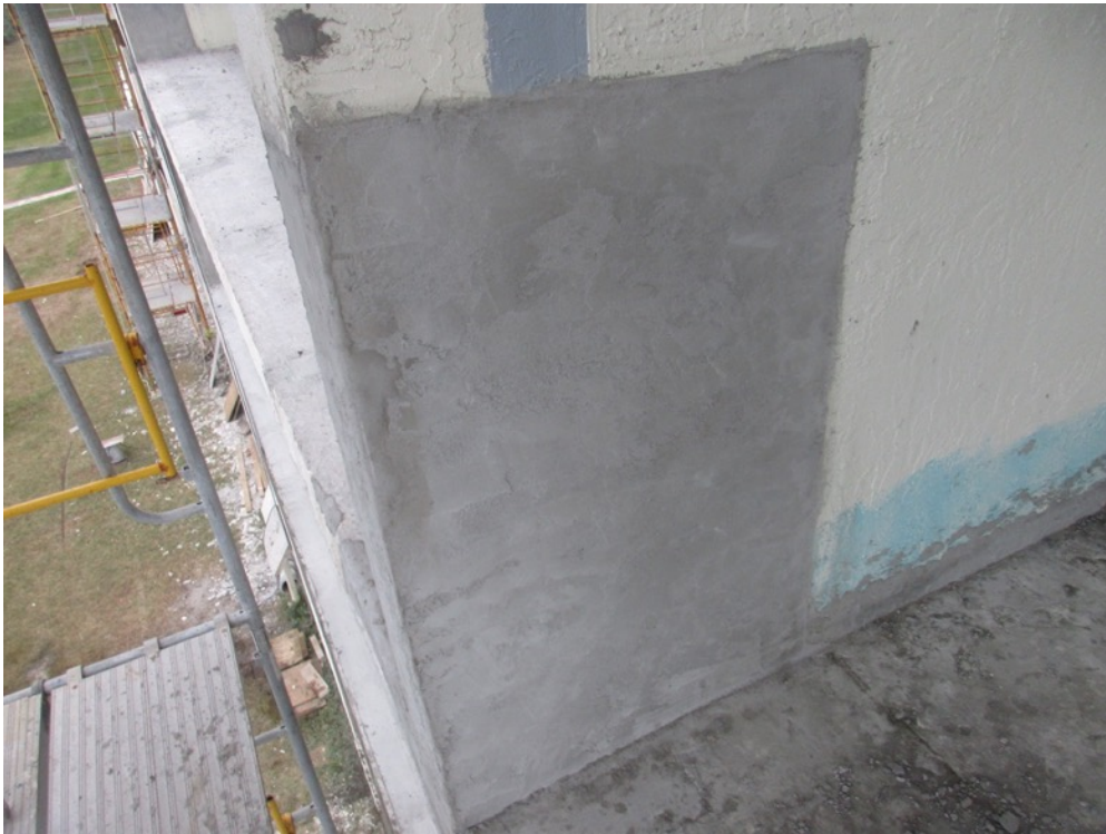
View of the Unit 231/232 column repair cast back with stucco finish applied
