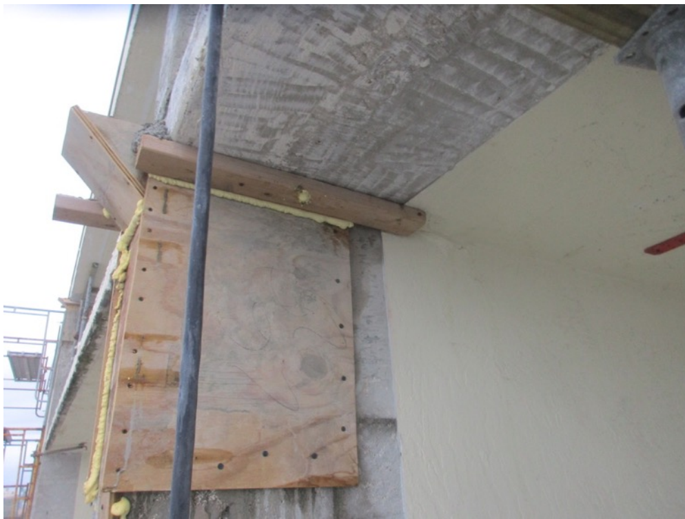
View of forms constructed with casting completed on the Unit 242/243 column repair
