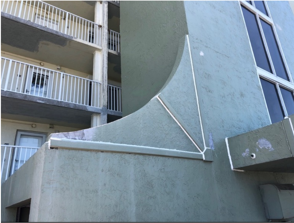
View of polyurethane sealant tooled at eifs trim perimeters on the west elevation exterior walls
