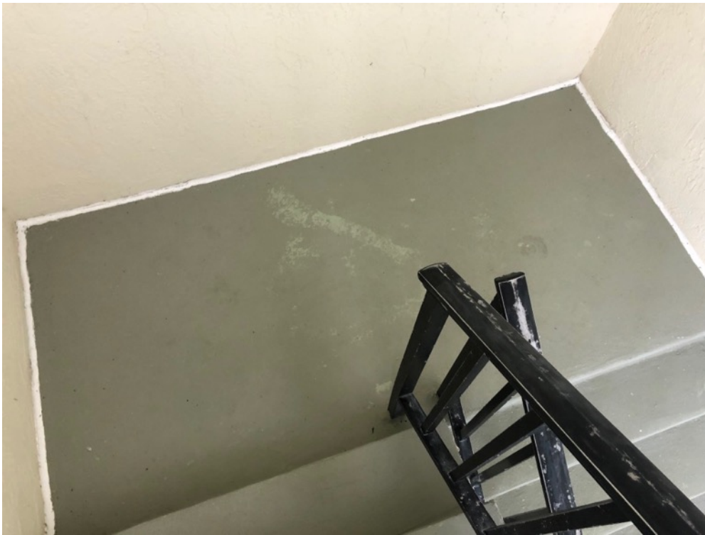
View of polyurethane sealant tooled at deck-to-wall juncture on the 5 th floor walkway north stair landing
